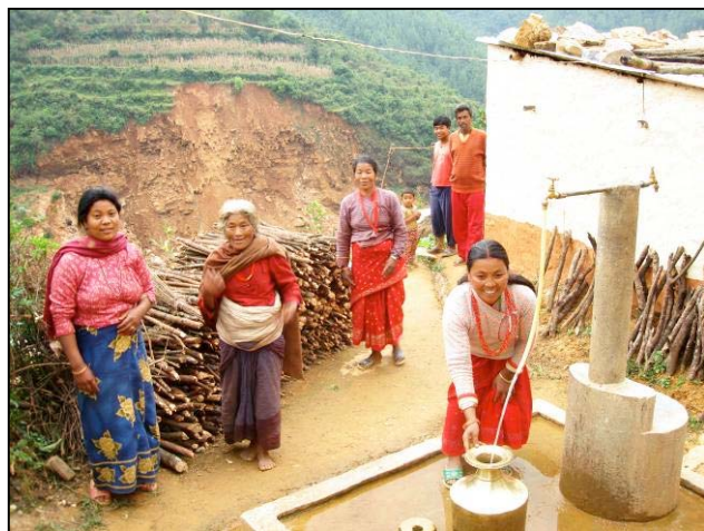
Multiple use water system (MUS) in Lalitpur District thru the USAID BDS-MaPS project. IDE has pioneered MUS in Nepal, MUS provide sufficient water for domestic use and for
